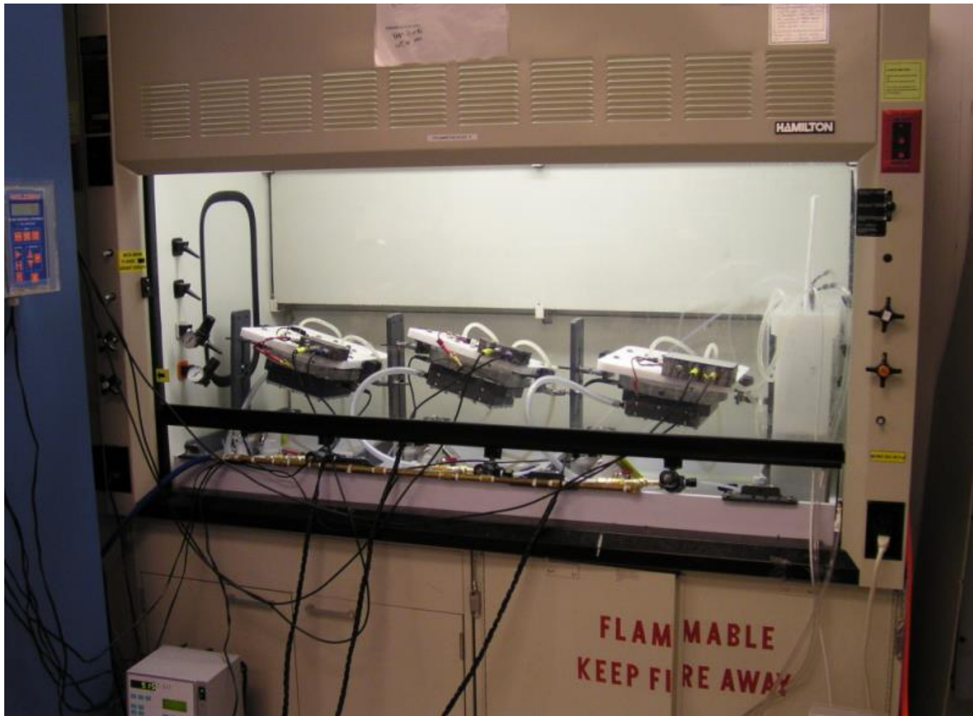
Installed System –Etching Cells Operating in a Hood
